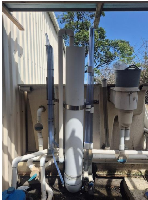
Figure 2 Experimental hydrostatic valve testing apparatus at CPA facility.
